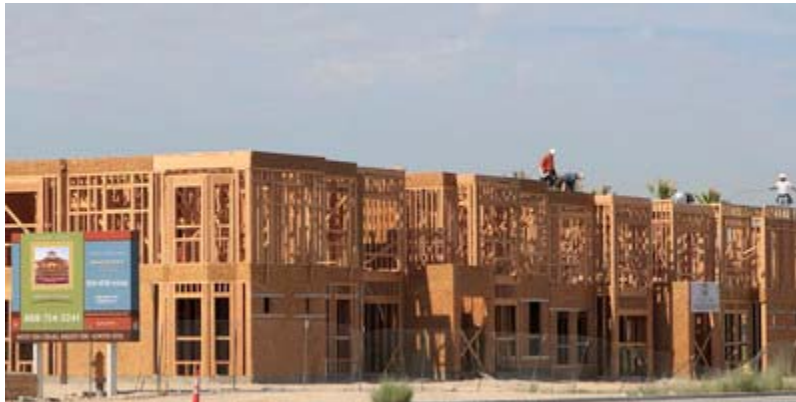
Sonata apartments at the corner of Craig and Lamb being built by Alliance Residential are seen Tuesday. Photo by Duane Prokop/Review-Journal
